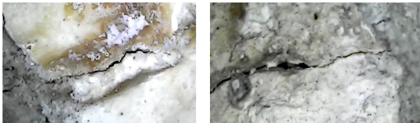
Fig. 8. Cracks in the structure (large scale)
