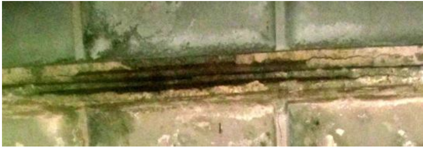
Fig. 1. Single cracks along the reinforcement on the edges of the ribbed floor slab
