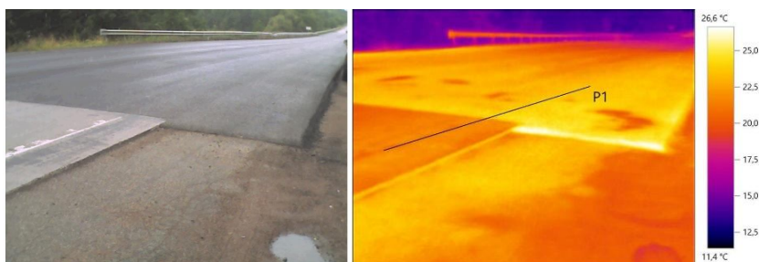
Fig. 9. General view and thermal imaging joint study of cement-concrete pavement with asphalt-concrete
